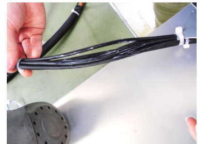
Cable unit A
